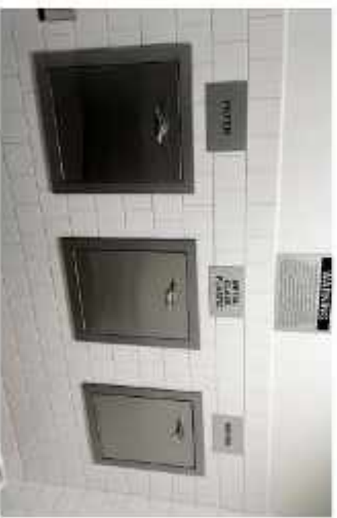
Three separate chute doors for trash, MGP and paper
