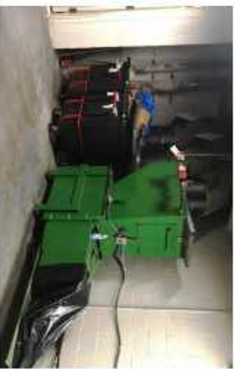
Trash chute empties into a compactor; MGP and paper chutes empty into 110L trash
